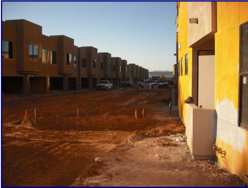
Above: the grading and paving for Phase 1 will be completed by November 1st.
